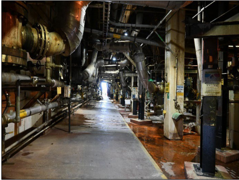
Figure 5. Interior of digester building.
